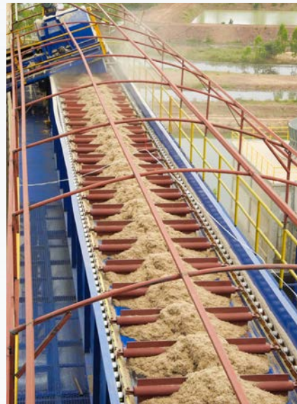
Figure 2-12. Drag conveyor carrying bagasse
